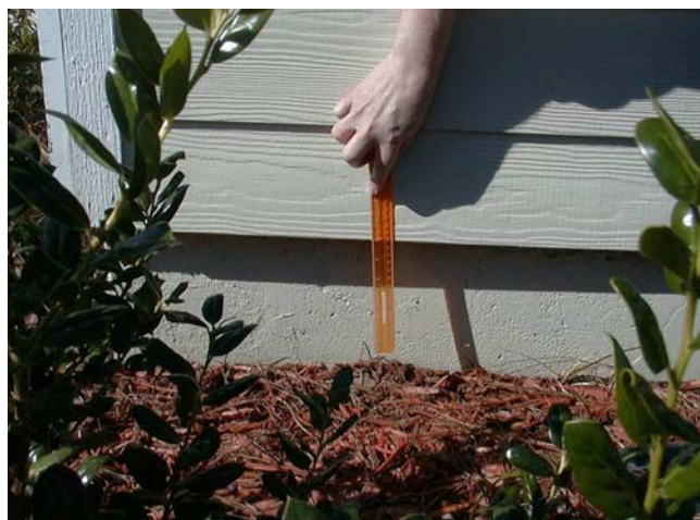
Figure 1. The current building code requires at least a 6 inch inspection gap, as shown in the picture above. The inspection gap between mulch and siding on the home will allow anyone to see if termites are building mud tubes into a structure.
