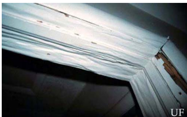
Figure 8. Blistered wood surface damage caused by the Formosan subterranean termite, Coptotermes formosanus Shiraki. Credits: Nan-Yao Su, University of Florida
